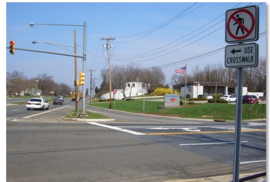
The existing crosswalk doesn't connect to the sidewalk (taken from the sidewalk)
